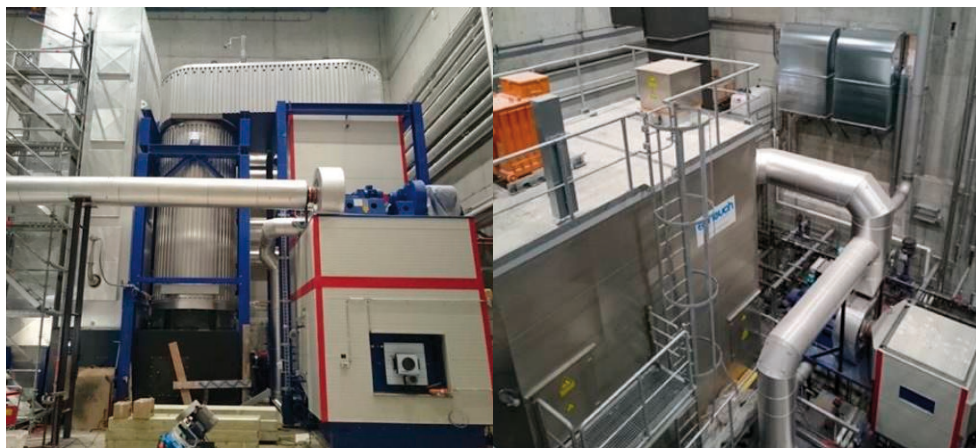
Wood chips and grain residues-fired boiler (KCO Kohlbach) with SNCR (ERC) (left) and electrostatic precipitator (Scheuch) (right) for process heat supply in the largest bakery in Switzerland. Photo by Verenum.
