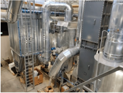
Tight emission thresholds in the NL require extensive flue gas cleaning at small scale district heating CHP plant: 2 x SNCR + cyclone + SCR + economiser + bag filter + condenser. Photo by ProBiomass BV.
